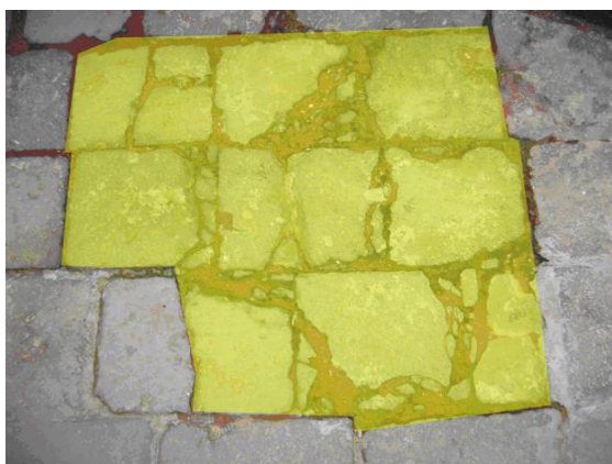
Dissesto in area ben delimitata
